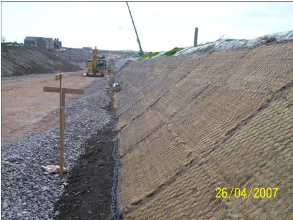
After Construction - the undulating nature of the cut has been covered up and regulated leaving an acceptable finished slope profile
