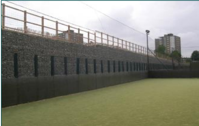
Gabion Noise Bund - Great Western Road, Glasgow 150m long and upto 5.5m high
