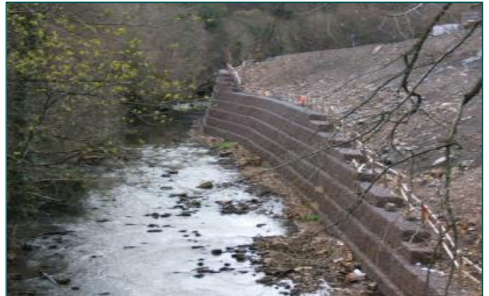
Eskmills, Edinburgh - During Construction 348m long, varying in height between 1.5m and 8m high
