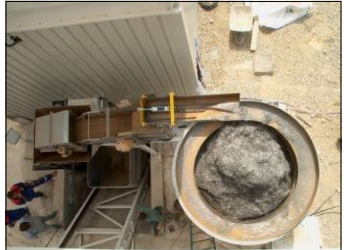
Maccaferri dosage machine attached to batching plant
