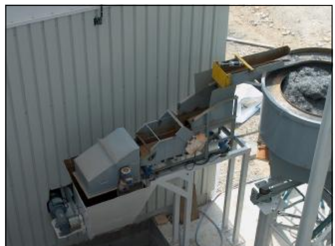
Computer controlled dosage machine at batching plant
