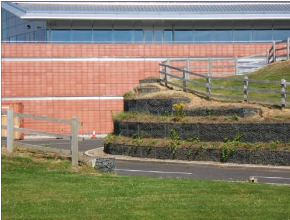
Curved Gabion Wall on either side of the access road - Under Construction
