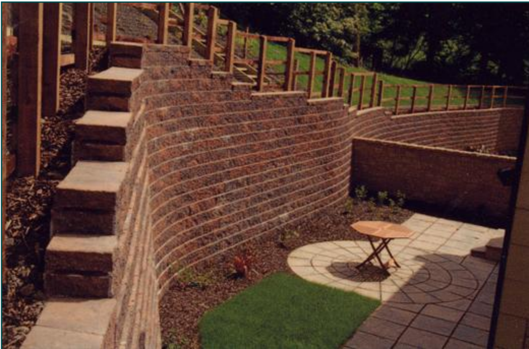
Balerno, Edinburgh - 85m long, varying in height between 1.0m and 3.8m high
