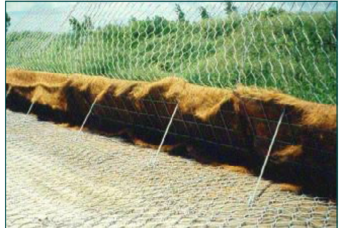
Green Terramesh unit (note factory fitted lost shutter, bracing angles and coir blanket) ready to receive backfill
