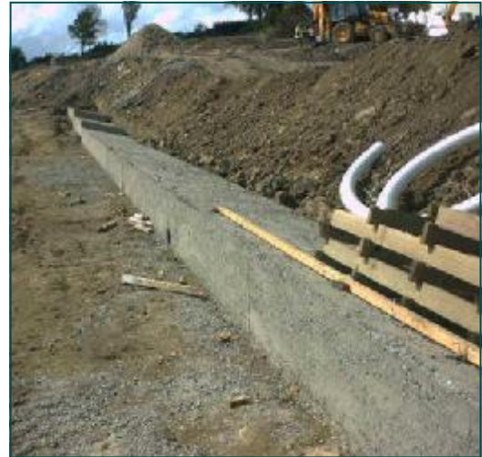
Concrete foundation ready to receive Timber Crib wall. The first course of timber headers can also be set into the wet concrete.
