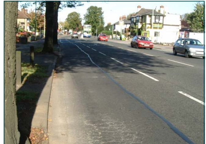
Before installation, showing fatigue cracking
